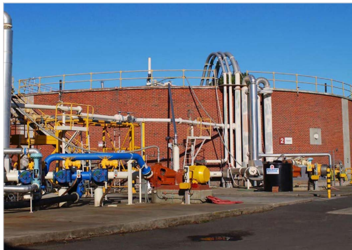
The sludge digesters deal with two streams of 'solids' – sludge from the primary tanks and waste sludge from the reactor/clarifiers (secondary sludge).
