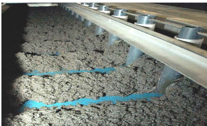
The gravity belt with thickened blended sludge.
