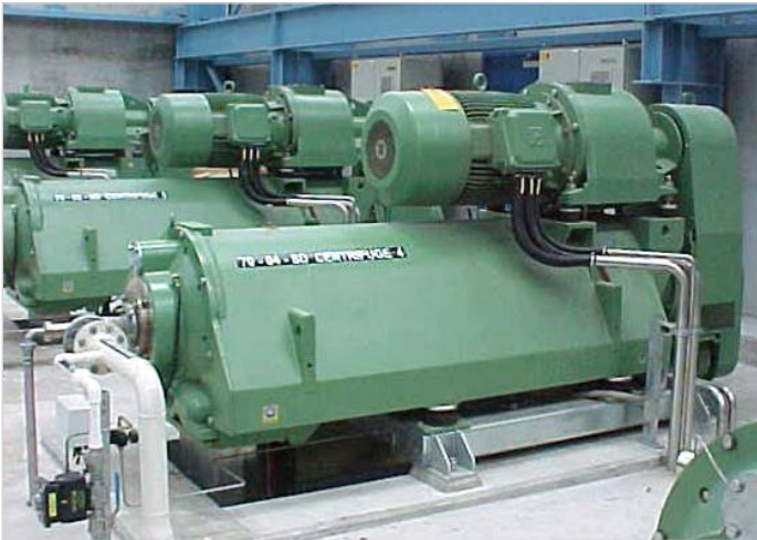
Centrifuges in the dewatering plant complex.
