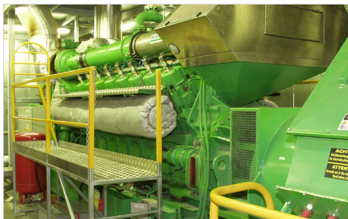
One of the four Jenbacher JMS 616 turbo-charged gas engine/generators.
